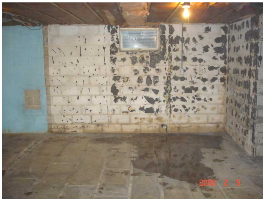
Mold and Mildew on the walls of a home
